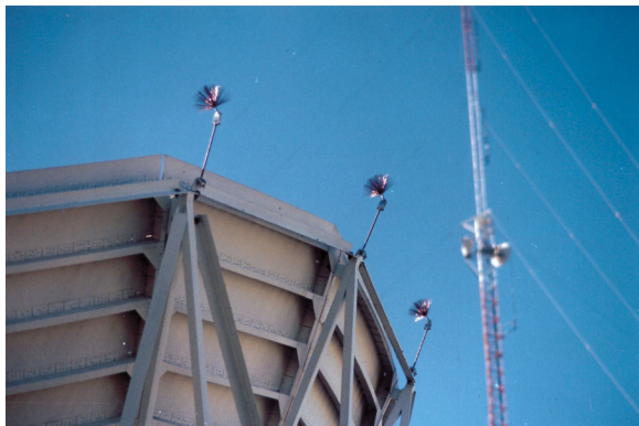
Lightning Protection on Dishes: A Closer Look
